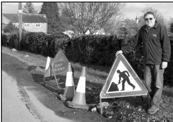
Barry has been working with residents at Whitecross trying to get a blocked roadside drain replaced
